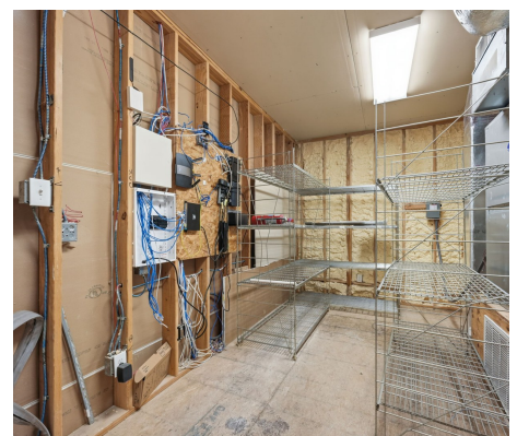
Mechanical / storage room
