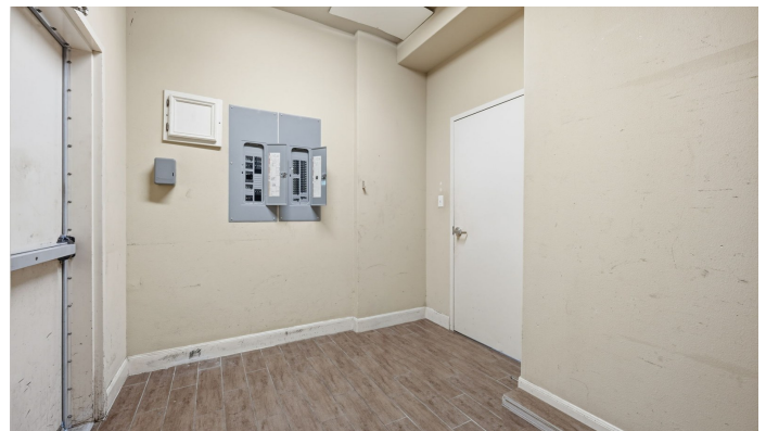
Storage room with electrical service
