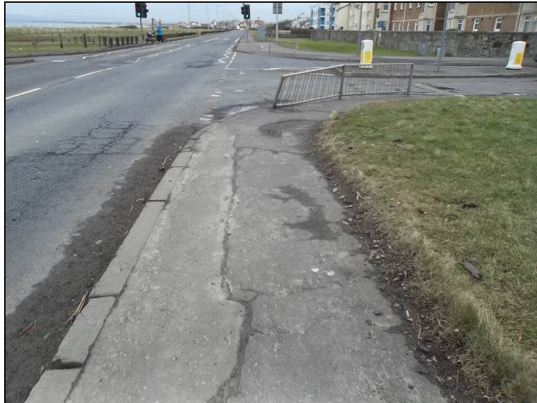
Footway along the eastern side of Beach Road looking north towards Burnfoot Avenue
