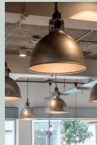
Spotlight lighting - ground floor
