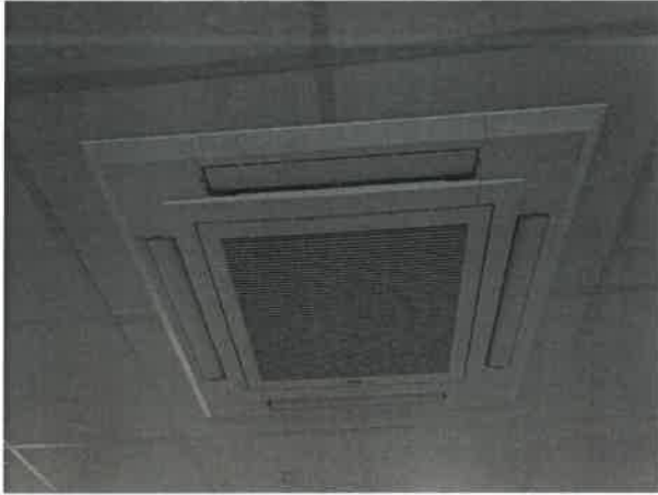
AIR HANDLING UNITS
