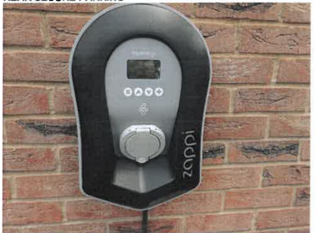
EV CHARGING POINT
