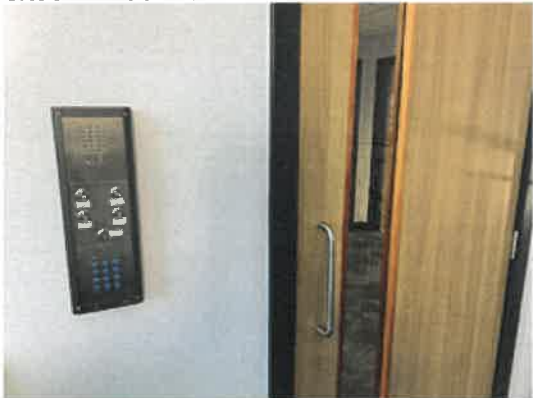
KEYPAD AND INTERCOM ACCESS
